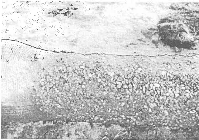
Fig. 20: Most slender section after cleaning. Upper pile has shown in fig. 19
