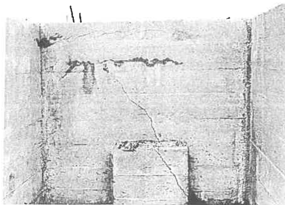
Fig. 2: Damaged r.c.-foundation beam, shortly after completion, due to excessive pile settlement
